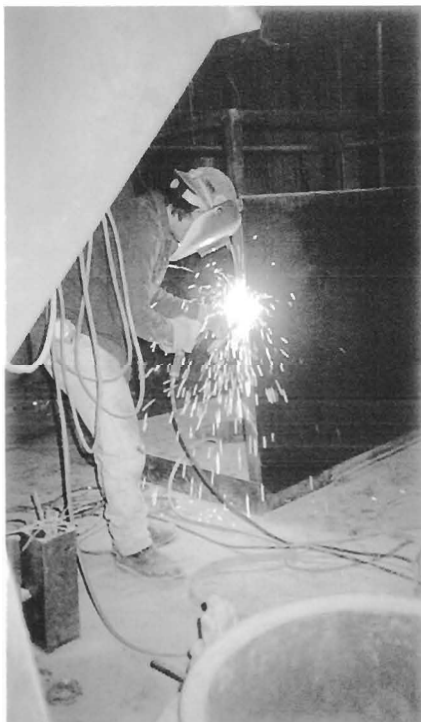
On-site fabrication assembly was carried out on the precipitator after an 18-week dismantling process revealed extra damage caused by the fire.
